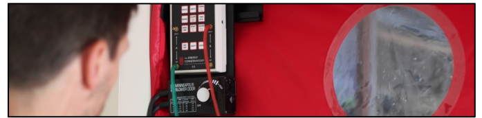
A red blower door, used by an Energuide Evaluator to seek heat leaks
